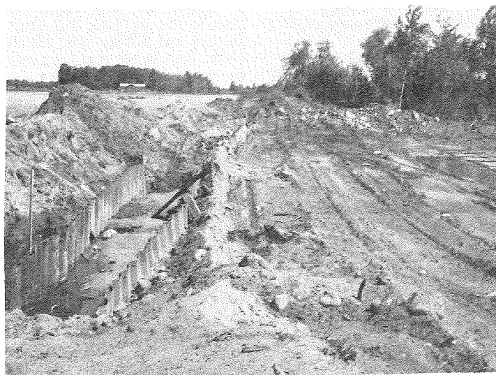
WORK GOES ALONG ON THE EAST SIDE OF THE MILLPOND-- Or beautiful Lake Weidman, where an emergency spillway was ordered constructed by authority of the DNR. As of Saturday, all the steel work was in, and work was beginning on hauling in gravel, stones and rocks. Messenger photo
