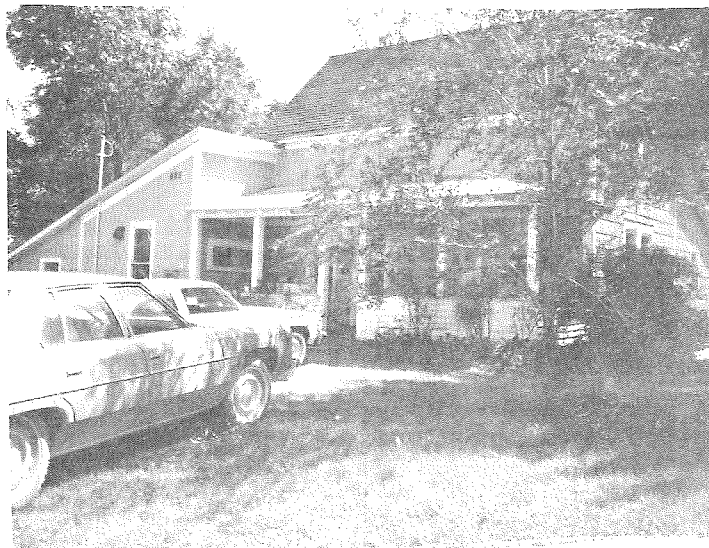
THE OLD ETHEL BYWATER HOUSE--Is undergoing renovation by the Dale and Sharron Sprague family of North Woodruff Road, who have purchased the property. Extensive remodeling and redoing are going on inside the house, with old plaster walls being torn off, ceilings being removed, all to be replaced by brand-new and attractive interior trim and finish. The job is no little one, as the Bywater house is one of the "oldies" in Weidman, and those oldies require nearly all-new interiors at least. Messenger photo
