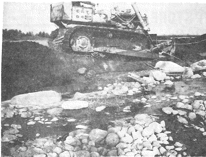
CUTTING OUT THE SPILLWAY AT LAKE WEIDMAN-- Tuesday morning completed the dam construction, begun last summer. A small bulldozer from Allen Lumber Company opened a channel at water's edge, and the spillover began, to lower the lake's water level in accordance with DNR specifications. (More photos on back page.)
