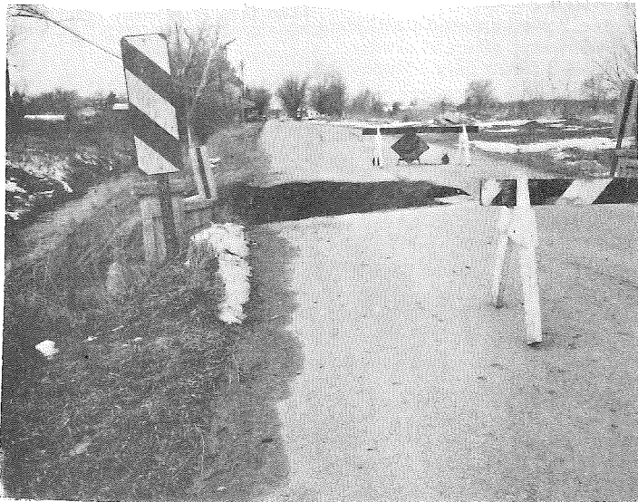
BRIDGE STREET TRAFFIC BLOCKED BY WASHOUT-- The bridge over the Yuncker county drain, east of the Bader Mill and the millpond dam, gave way Monday morning, and all traffic was re-routed to enter Weidman on East Weidman Road, go through the main business street, and finally hit the Airline Road. It will be some time before the bridge can be rebuilt, as extensive damage was apparent, necessitating the rebuilding of the entire under-road cement structure. Messenger photo
