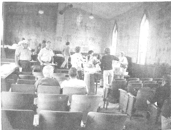
THE INTERIOR OF THE SHERMAN CITY CHURCH-- Is in surprisingly good shape, considering the many, many years of neglect, vandalism (all the windows are broken out) and just plain disuse the church has endured. Church officials feel that the floor is solid, the theater-seat pews will do for the nonce, the good wood wainscoting will be sanded and shellacked, the walls and ceilings (the latter with some repairs) will be scrubbed and possibly painted. Otherwise, the interior is good, it's solid, it's usable. It's a miracle, after all these years.
