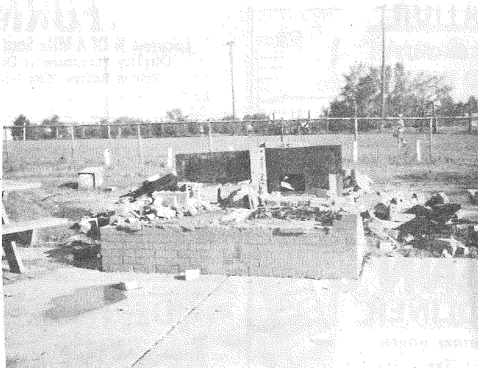
THE HUGE BRICK FIREPLACE AT THE PARK --Real favorite of vandals, has been obliterated, readying space for the new community building. The new building is expected to be completed before bitter cold sets in.
