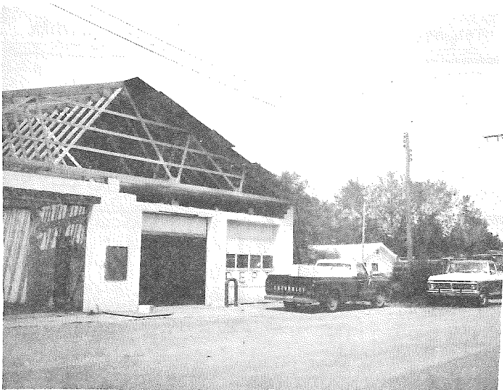
HERE'S A CLOSEUP-- Of the front of the Fire Hall as of Friday. Work was expected to be completed Saturday. Jerry Straus is contractor for the job, with Volunteer Firemen putting in endless hours working with him on the roof.
