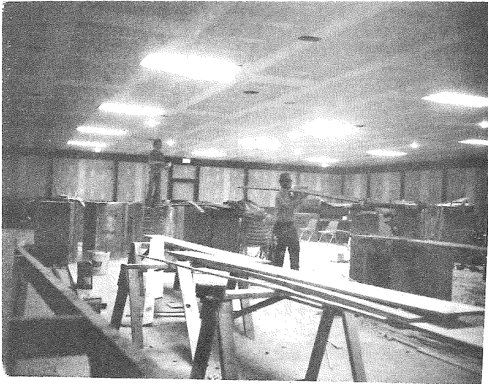
WORKMEN ARE FINISHING-- The inside of the new Community Building in Mitchell Memorial Park in Weidman. They're working on side walls, and next will be floor finishing. Weidman Business men plan to paint the floors of the huge building.
