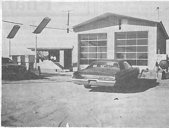
RAY'S SERVICE STATION TAKES ON MODERN REBUILDING-- Ray Battleshaw's service station at the corner of Weidman and Woodruff Roads--the entrance to the village of Weidman--has been undergoing dramatic changes, with an old section torn out and a 30x40-foot new garage building attached to the remodeled office space. Messenger photo
